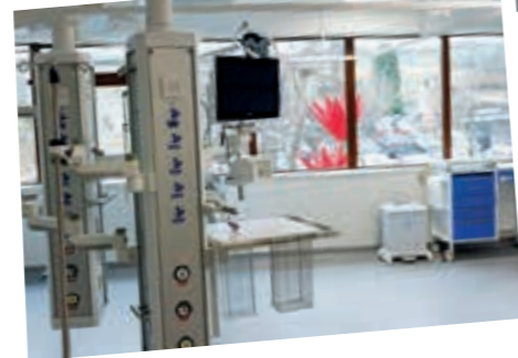
Top: The new pendants provide 360-degree access to patients around the bed.
